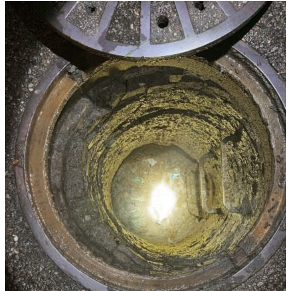
Grease blockage in a manhole caused by apartment complex, likely from disposing by pouring kitchen fats, oils an grease down the drain.
